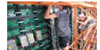
Difficult to maintain, High maintenance costs
